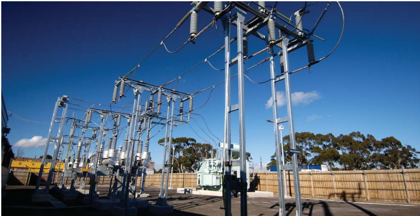
a typical zone substation
